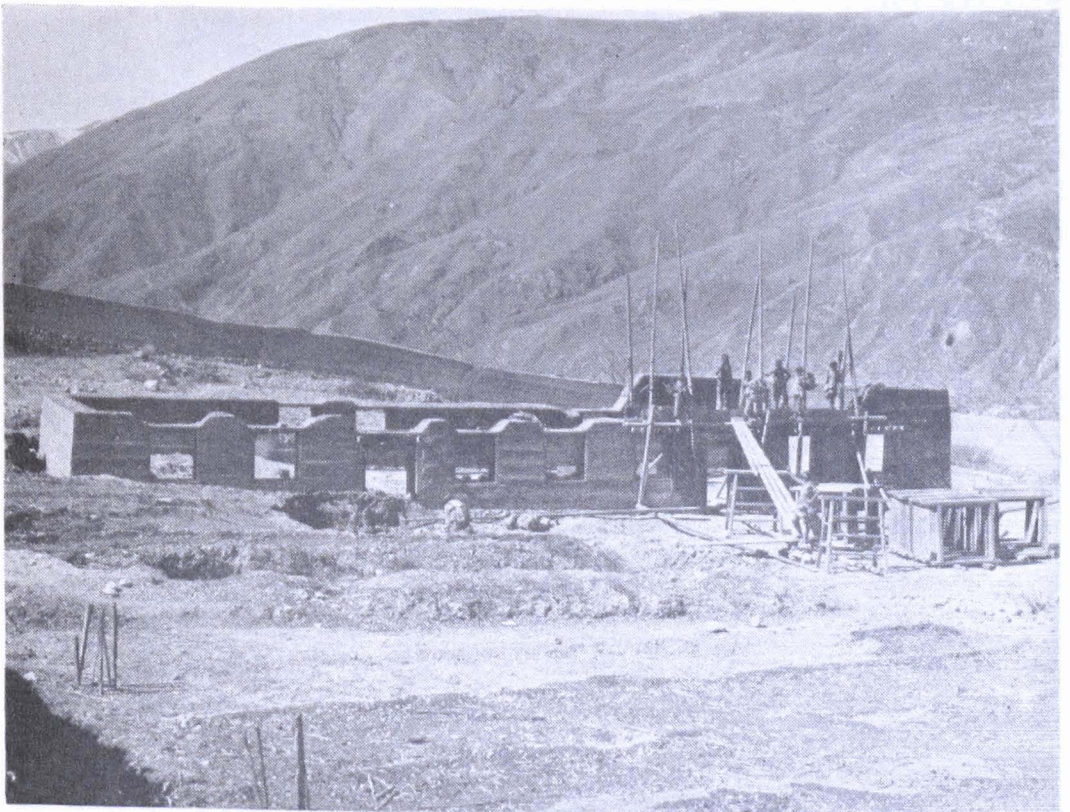
PLATE 9. The walls slowly rise around the doors and windows which are prepared by carpenters beforehand. This is the orphanage building at Batang.
